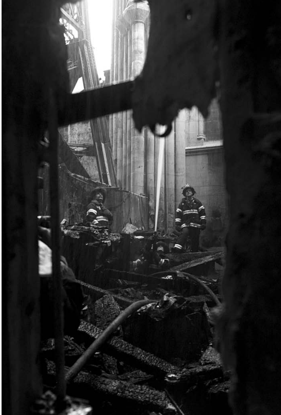
Figure 3 A view of the interior of the north transept after the fire. Charred wood beams and partially melted bituminous materials from the roof structure are in piles on the floor. (Michael Schwartz/New York Daily News)
