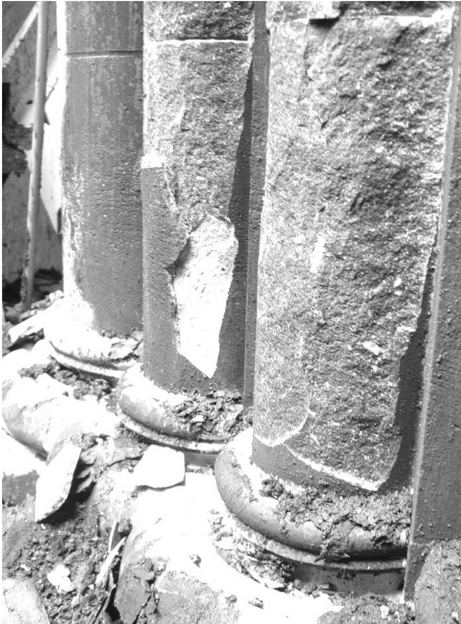
Figure 4 The limestone in the north transept exhibits spalls from the stresses caused by the heat from the fire followed by sudden cooling when the water used to extinguish the fire hit the stone. The stone was blackened by the deposition of smoke, which was heavily laden with bitumen.
