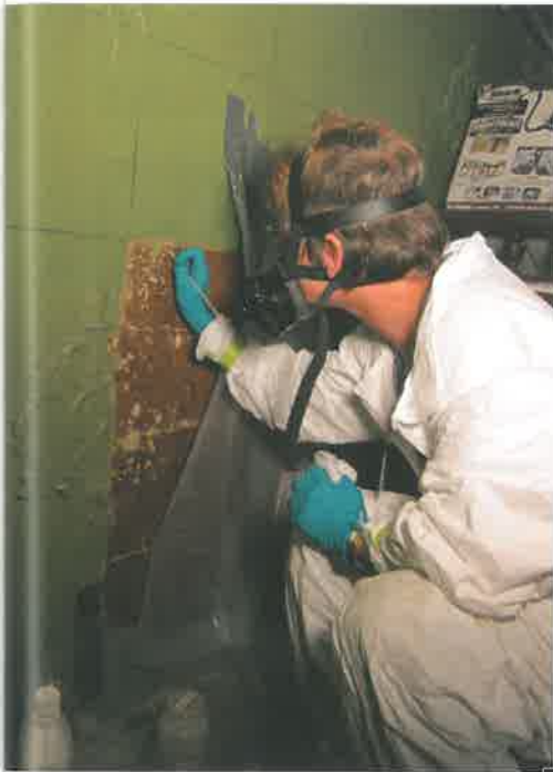
Fig. 9. Company Room D, showing Melissa McGrew of BCA testing non-proprietary paint removal formulations on the wall, 2010.
