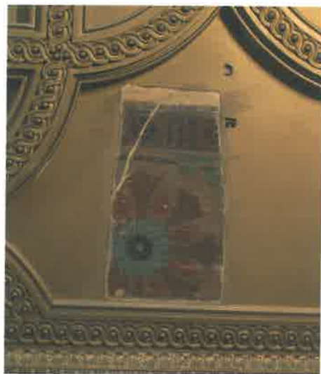
Fig. 3. Portion of Company Room D ceiling. Cast-plaster panels had been nailed over the original 1880 painted finishes. Here, several of the panels have been removed.
