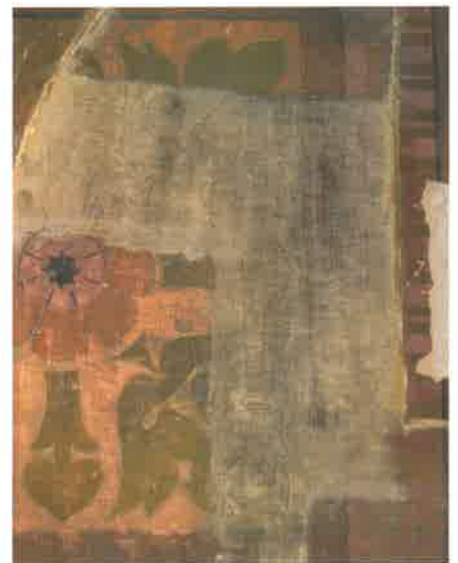
Fig. 10. Company Room D, detail of ceiling, 2011. Overpaints were only partially removed. At the bottom half of the image, the surface is unvarnished, and overpaints are visually distracting. The top half of the image is the same surface but with a varnish applied to it. The overpaints are still visible, but the impact is muted by the saturation of the colors that comes with application of a varnish.
